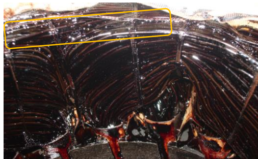
Fig. 10 Sample 3 End-Windings After Failure. Phase-phase overlap in the EW region is highlighted
