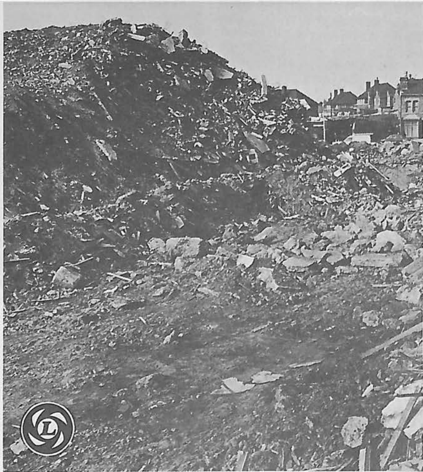
British Leyland's van plant at Adderley Park, Saltley. Closed in 1972 the site is now being redeveloped as a warehousing estate and lorry park by a Wimpey's subsidiary. But new tenants are hard to find — so far there is only one.
